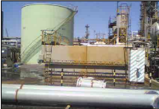
Basin in petrochemical complex
